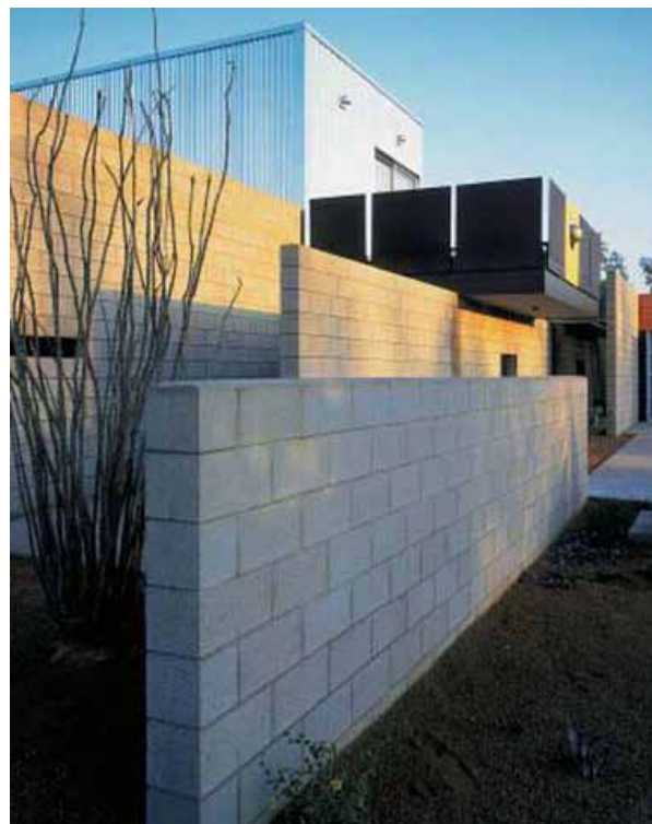
Figure 2—Effect of Changing Sunlight on Gray Concrete Masonry
